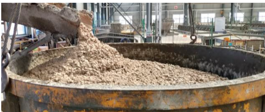
3 The concrete transfer from mixing to pouring for the precast ribbed wall panels
