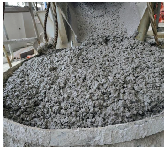
4 The concrete transfer from mixing to pouring concrete for the precast tunnel segments
