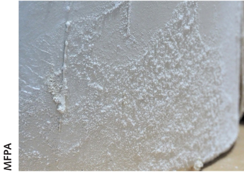
5 Crystallisation of sodium sulphate on the outer surface of a gypsum mould
