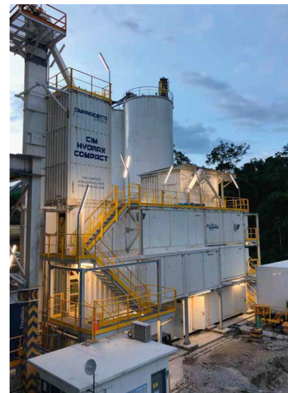
12 Hydrax COMPACT lime hydrator in a plant in Colombia
