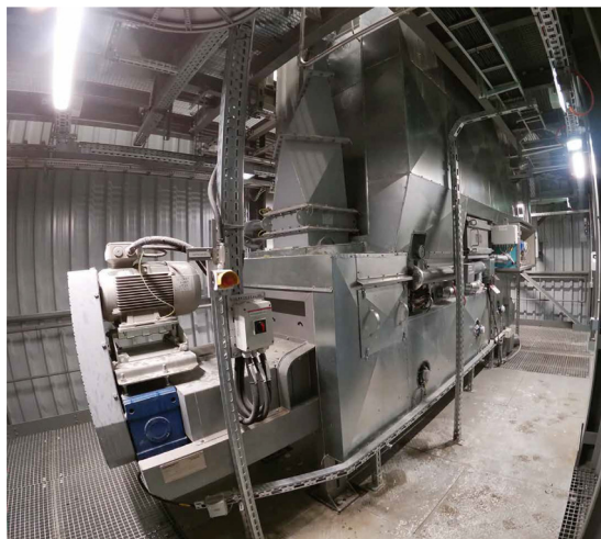
17 Hydrator in a waste-to-energy plant in Europe
